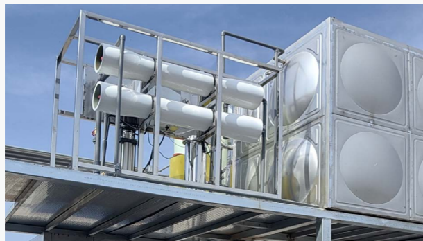
· Milk Collection Center Wastewater Recycling Project ·
